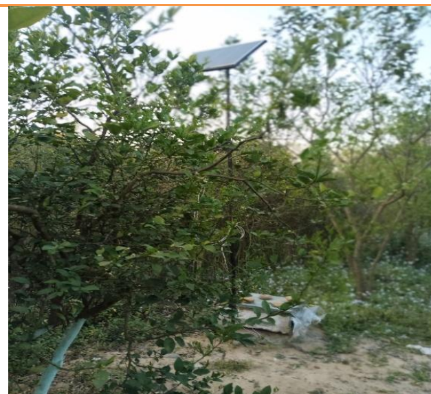
Figure 1 solar powered light
